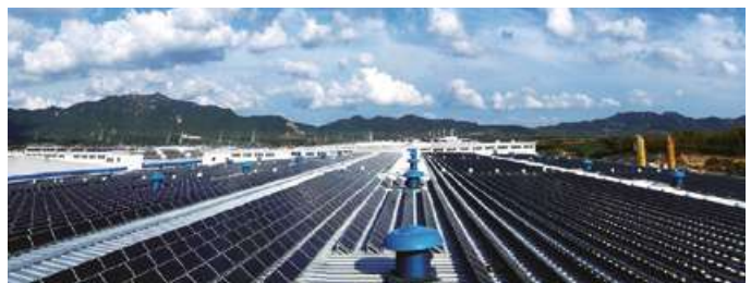
Solar panels arrays
